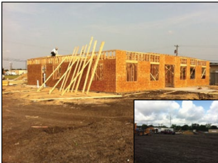
The Texas Mid Coast Chapter makes great progress in the building of their new offices/training facility. The new building is slated for a 2013 third Quarter completion.
